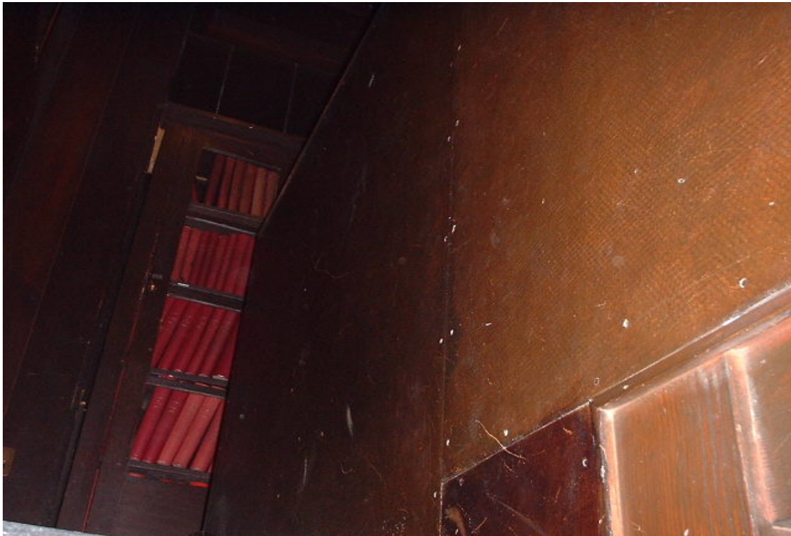
Asbestos Cement Boards @ Library Stairwell
