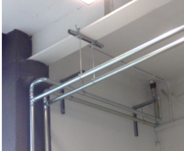
Fig.5 – Typical heating installation pipework in the studio spaces.
