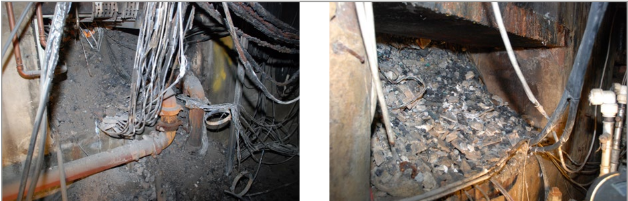
Figure 19 – Cables exiting vertical ducts into level 2 Plenum
