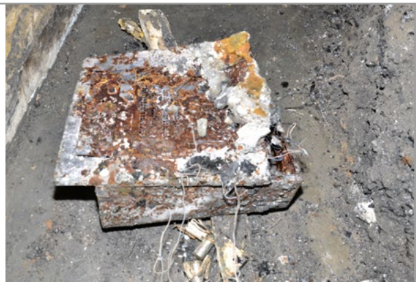
FWS control panel prior to impounding
