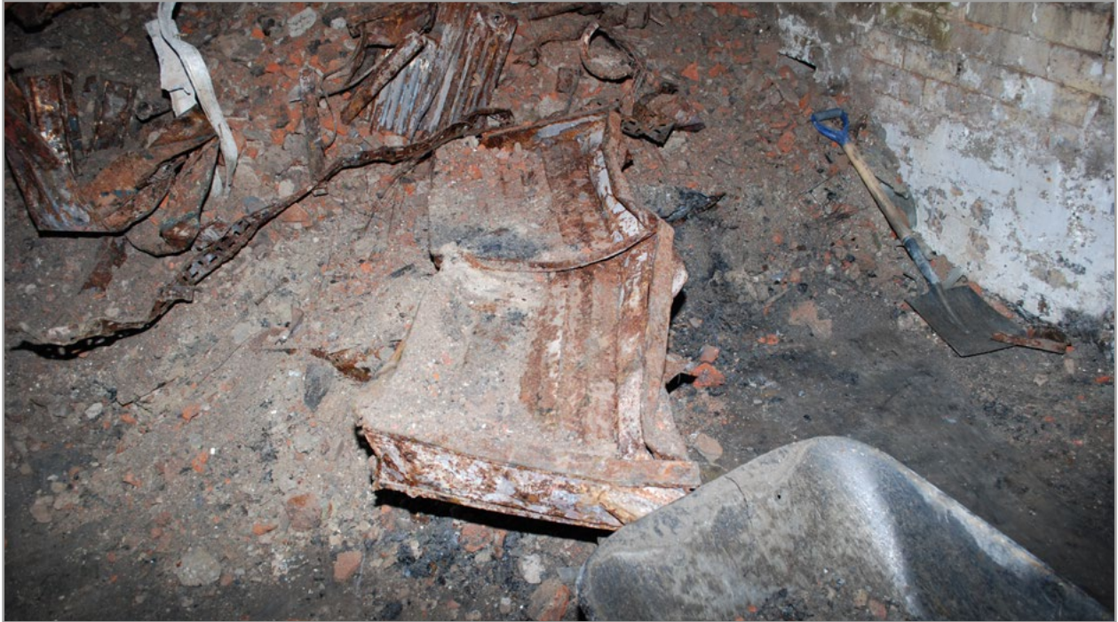
Figure 16 – Metal duct work installed in level 6 plenum, found on level 2
