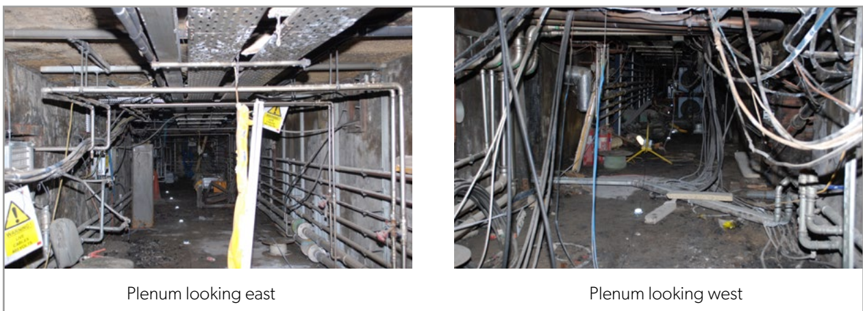
Figure 18 – Plenum below level 2
