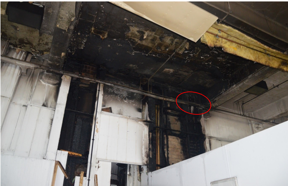
Photo 13. Ground floor studio 31 west side. Fire spread up each vertical void. Suspect fire spread to these voids horizontally from the left. Circled area horizontal void leads to studio 32.
