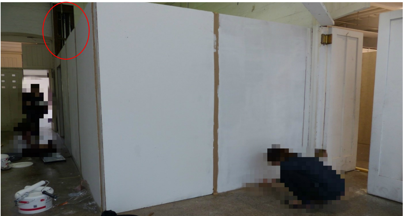
Photo 27. Exterior image of the student display area within studio 19. This was taken two to three days prior to the fire. Note the area circled is the pipe void with panels removed. Image courtesy of Police Scotland.
