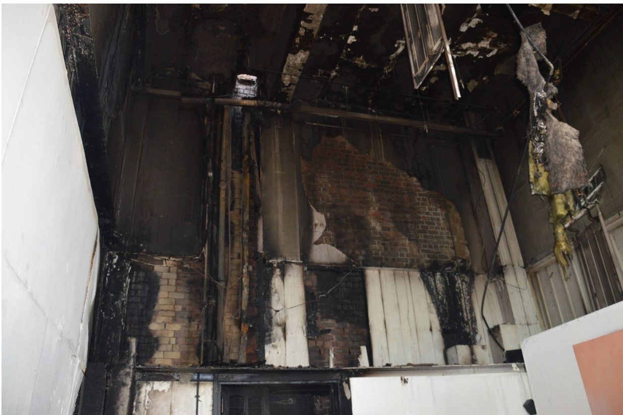
Photo 17. First floor studio 44. Looking south, fire spread up vertical voids to 2 nd floor
