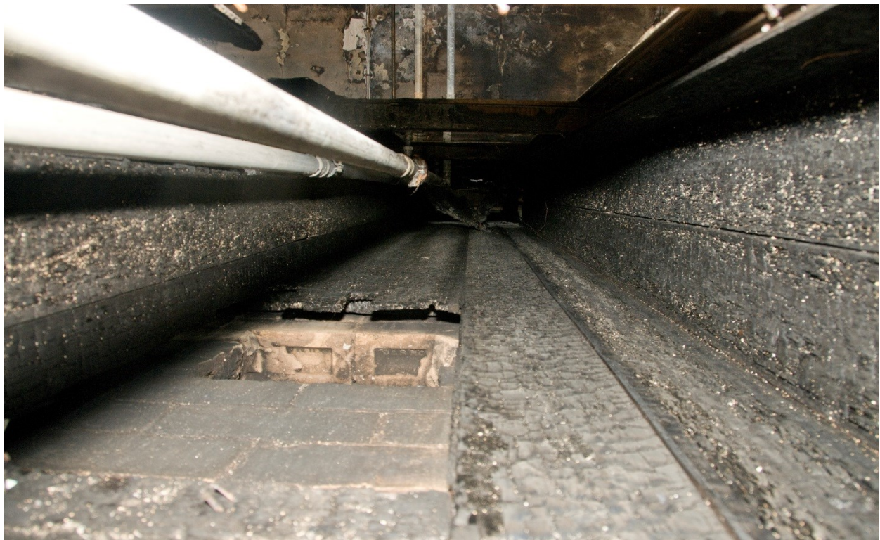
Photo 9. Void running from basement studio 19 to roof
