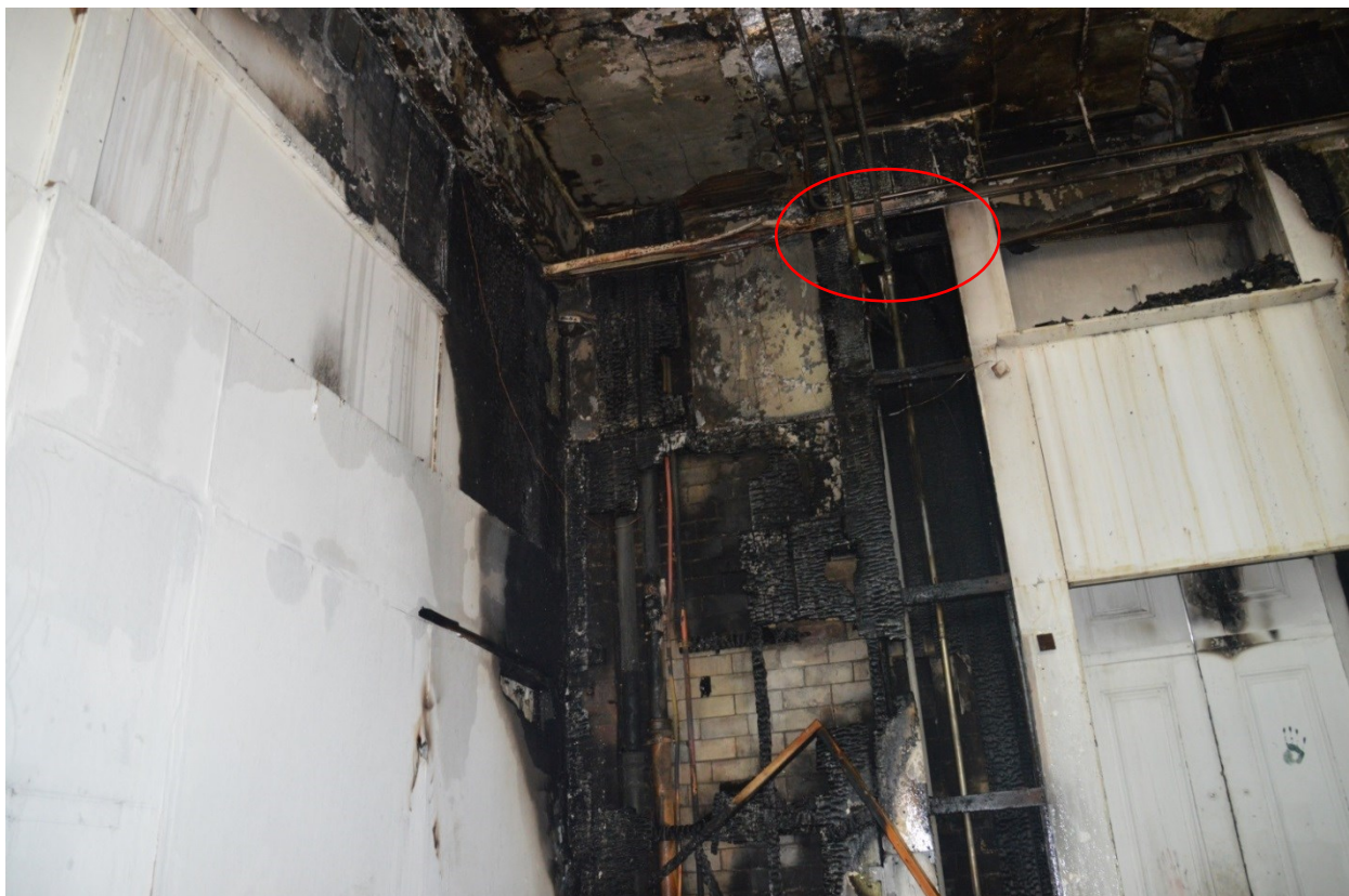
Photo 11. Studio 31 Ground floor. To left of door, fire spread to first floor via void area circled.
