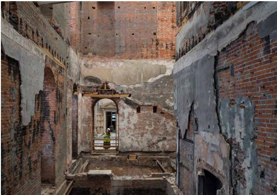
Clandon Park, post fire
