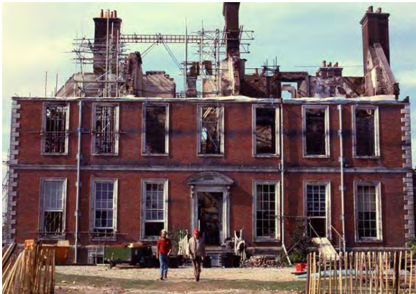
Uppark House, fire damaged
