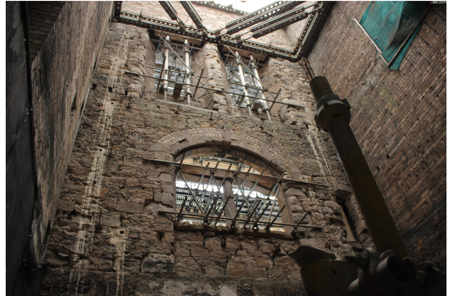
Internal view of windows on this front indicate the level of instability and missing window panes
