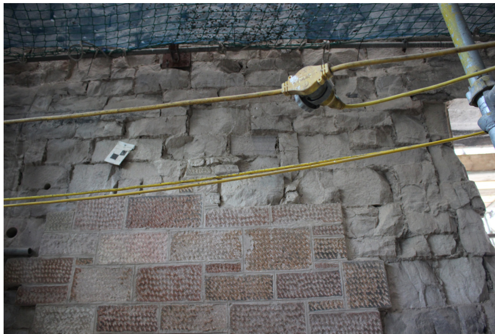
Pilot scheme of resurfacing illustrating damage internal stone face.
