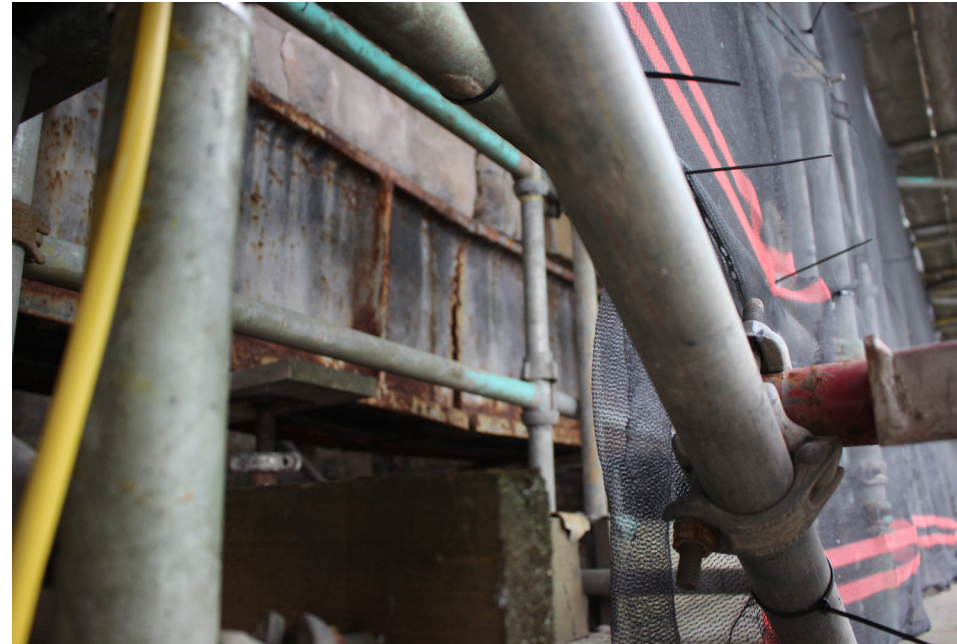
Crack in iron girder caused by fire
