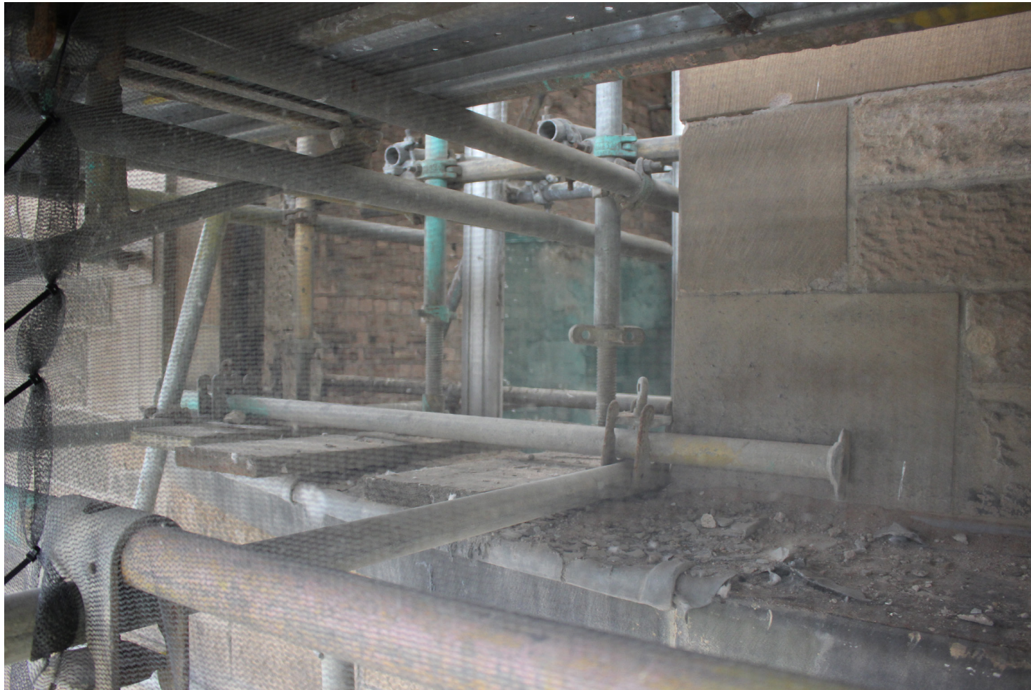
Missing window frames on east front fenestration
