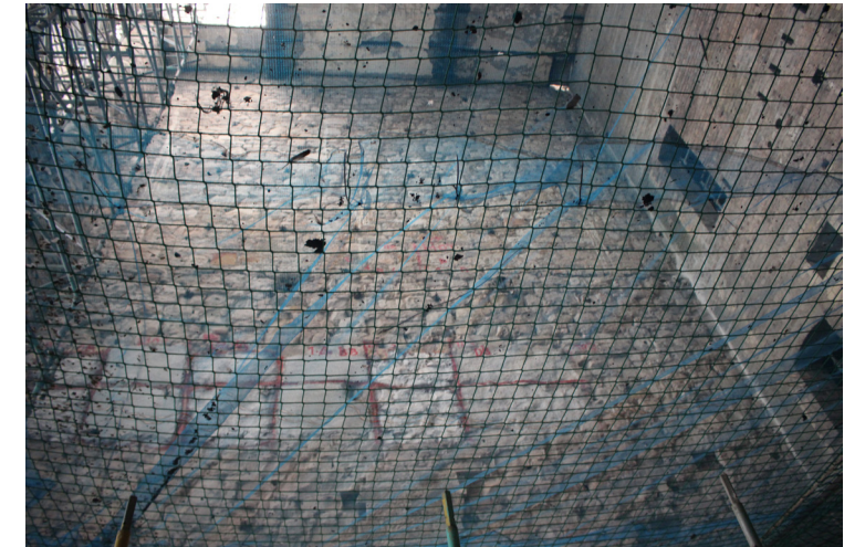
Missing floors inside site with visible doorways and mortice holes
