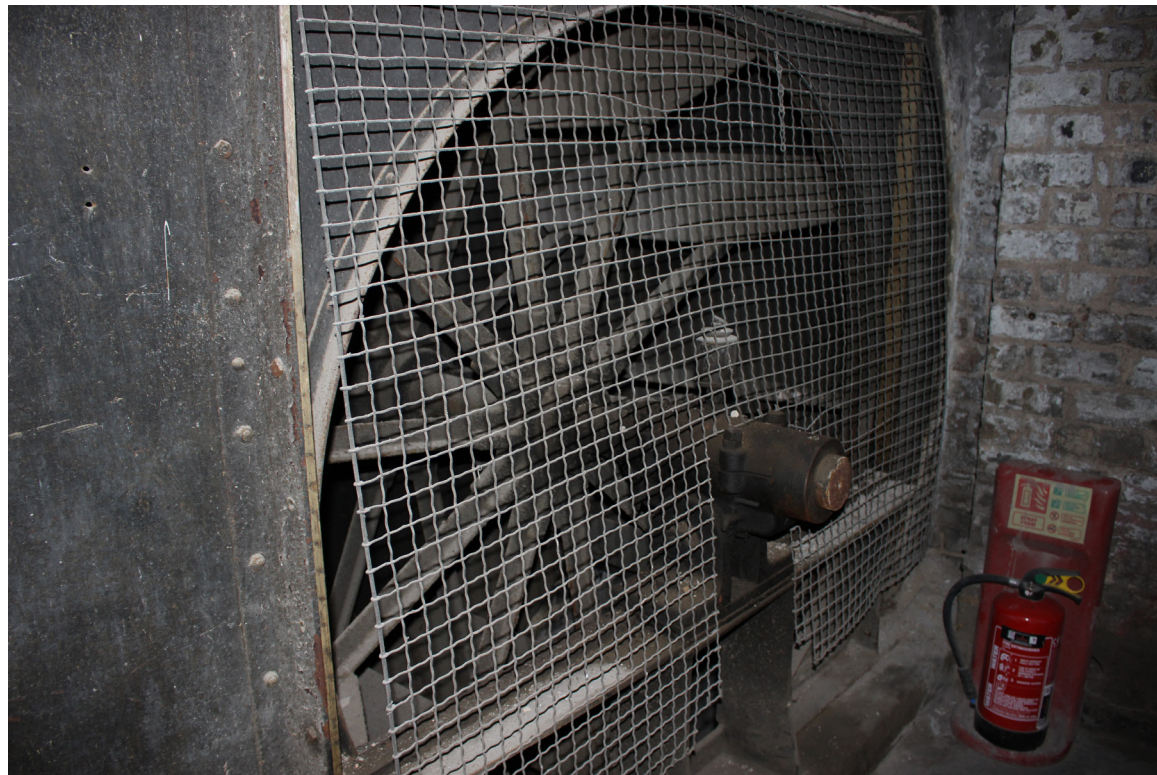
Historic heating turbine which survived fire and remains in basement
