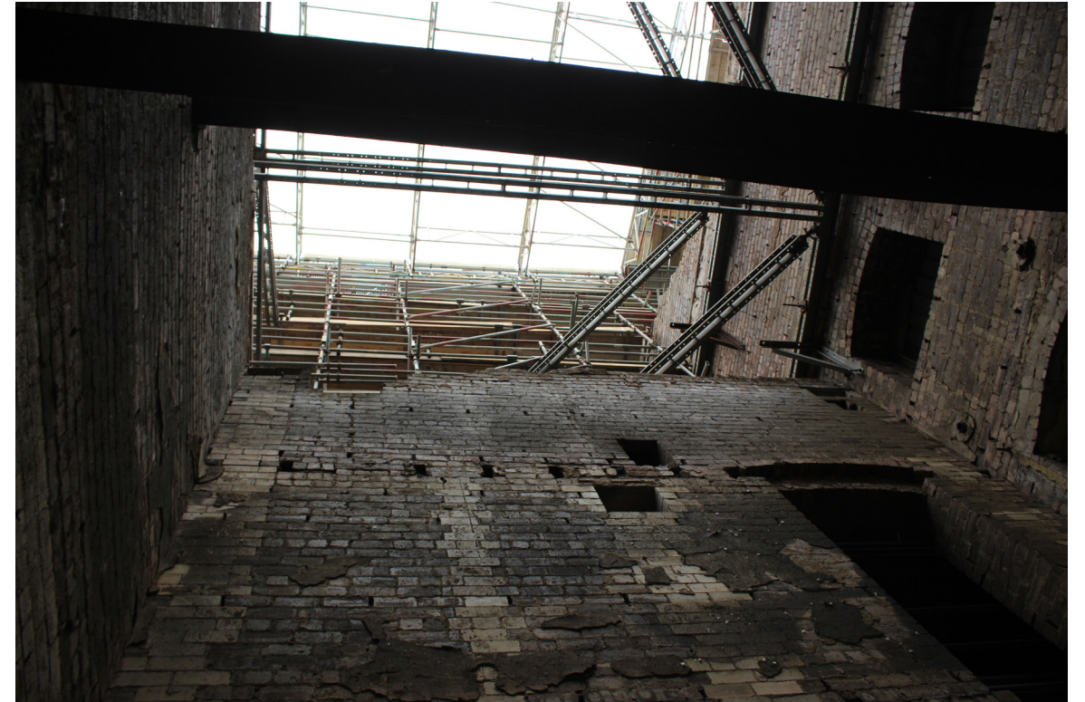
Damaged brick work in central bay of southern section
