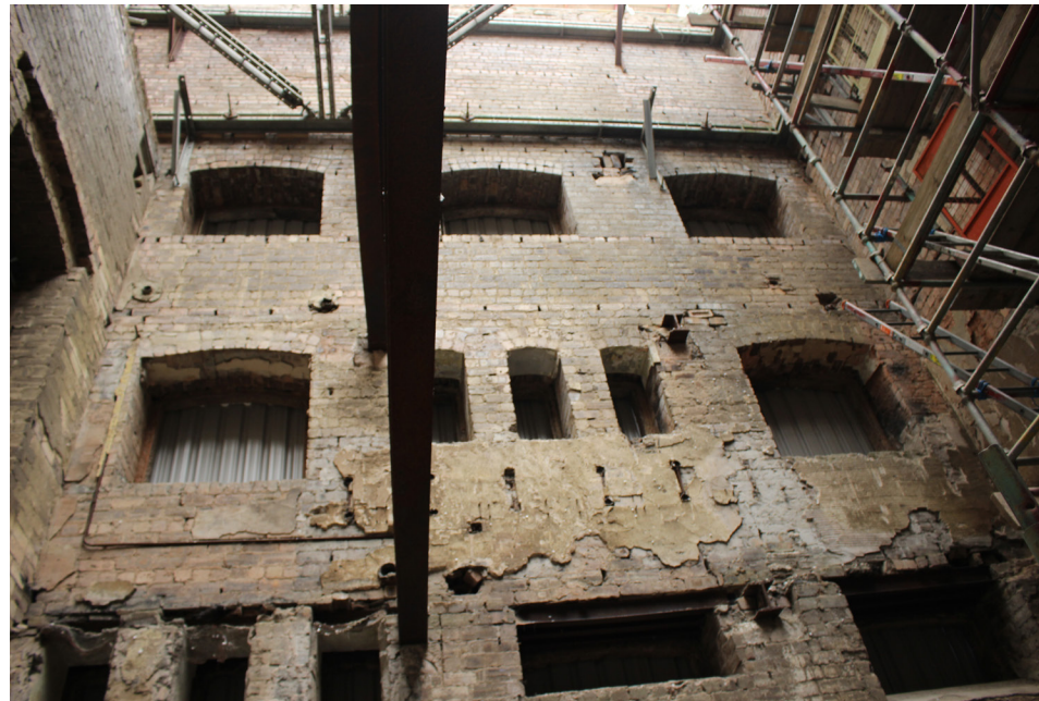
Blocked over fenestration in south front
