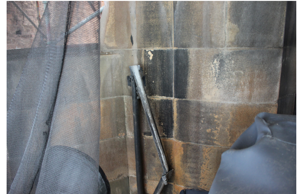
Melted metal work and scorch marks from fire on north front
