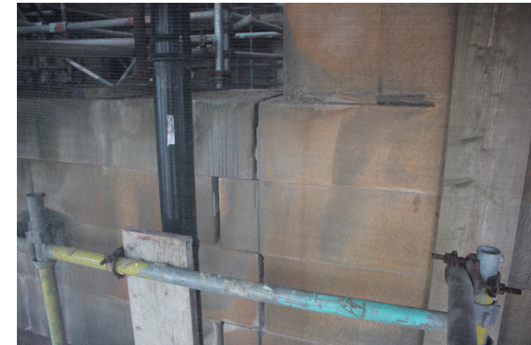
Movement in masonry causing separating blocks on west front
