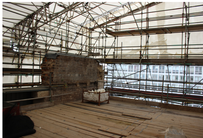
Missing ornate fenestration on western front.
