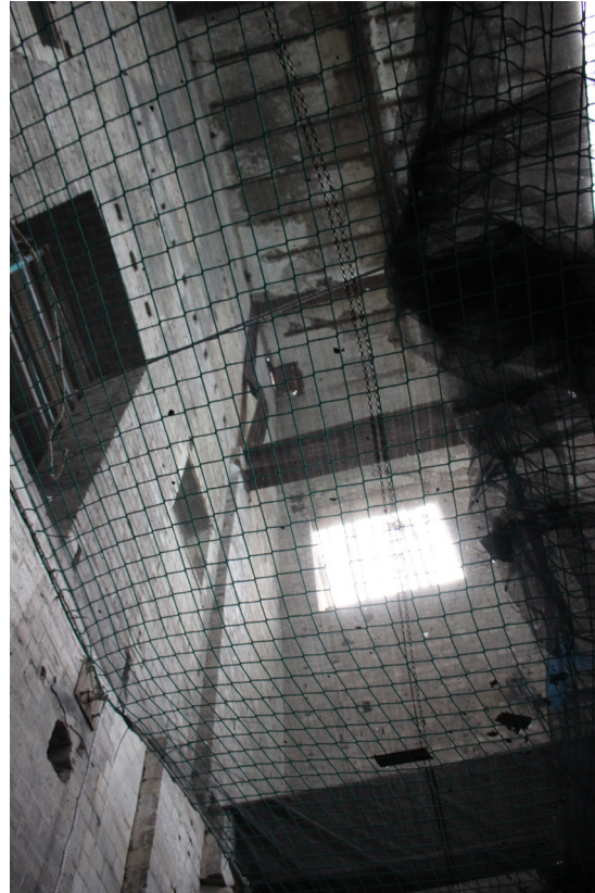
Fire warped girders spanning width of room
