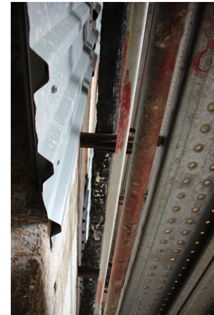
Burnt 12m long timber beam in courtyard
