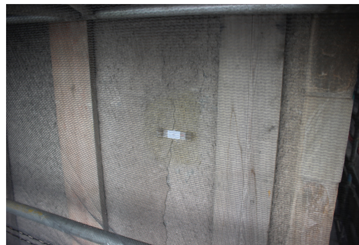
Crack through on south front being monitored for movement
