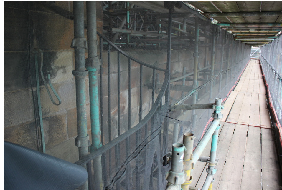
Balcony railings survived fire
