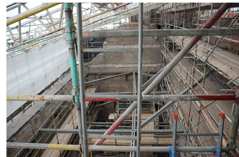
Burnt out shell of central protruding bay on the south front with sloping missing roof.
