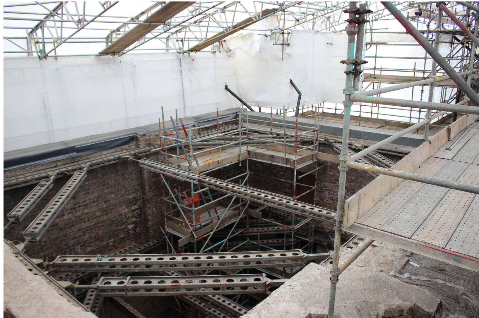
Southeastern most bay with missing floor and scaffolding supports.
