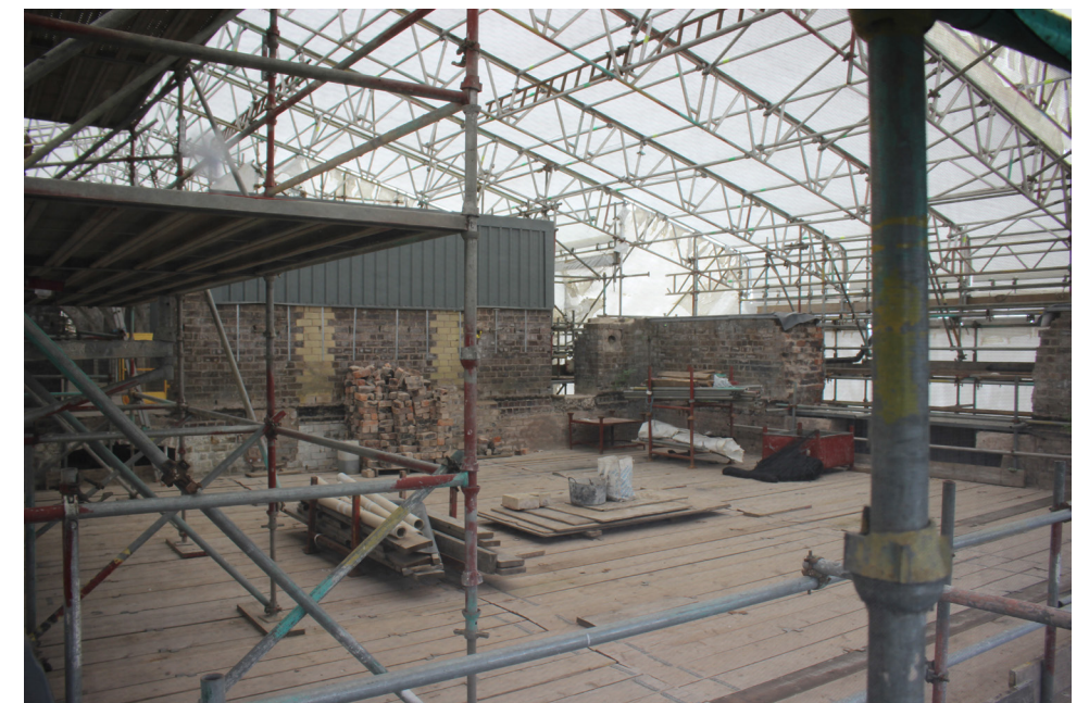
Broken walls on western end of roof, large opening to right was the once prominent decorative south facing window
