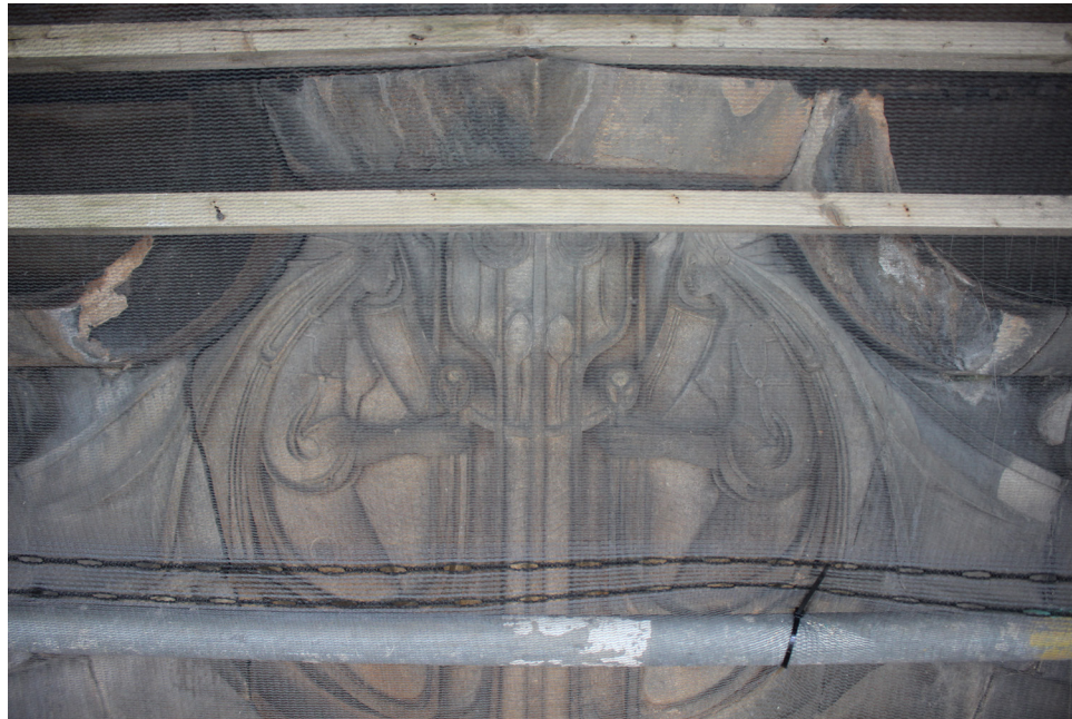
Guardians badge suffered minor damage from fire
