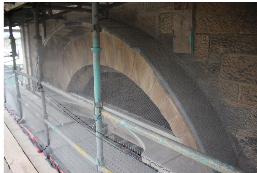
Decorative arched moulding on east front has suffered minor damage
