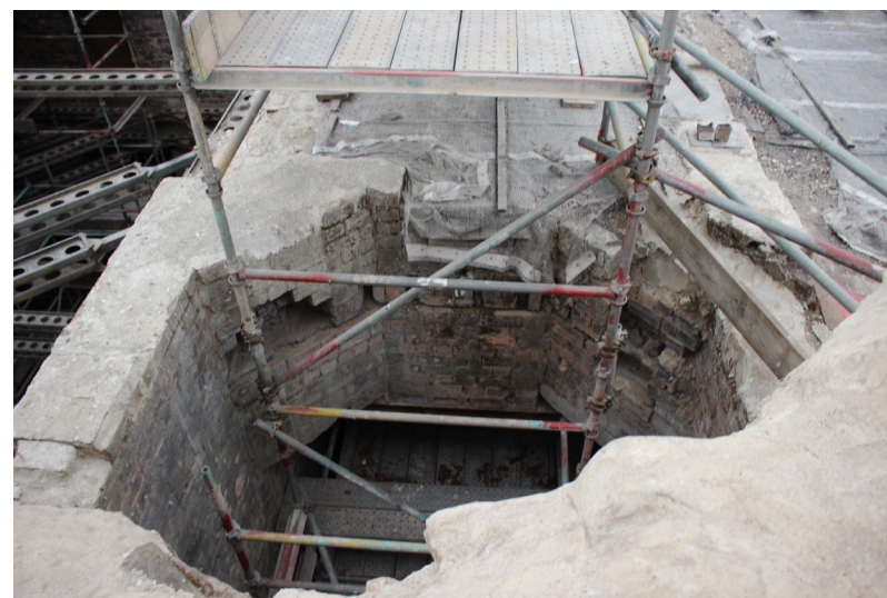
Burnt out turret on roof
