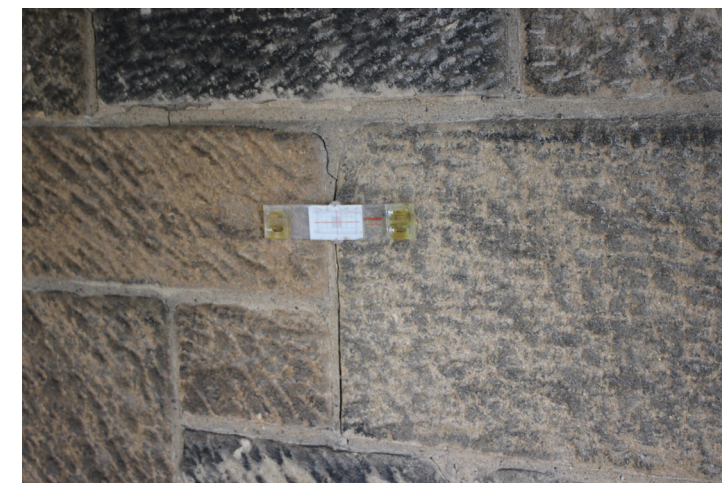
Movement in masonry of building, masonry fused with molten lead
