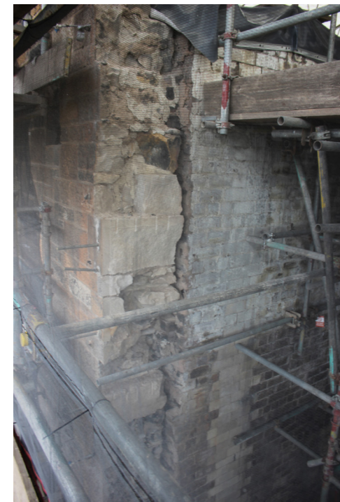
Separation of external masonry with internal brick partitions along north front
