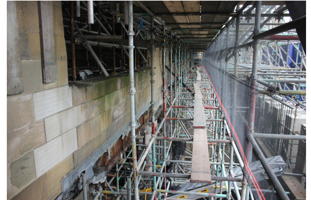
Void space between street and north front showing missing basement roof
